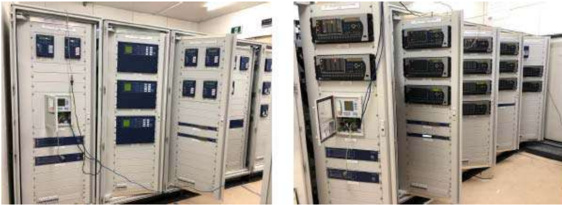
Figure 1 – Control Room Protection Panels Commissioning at Substation
